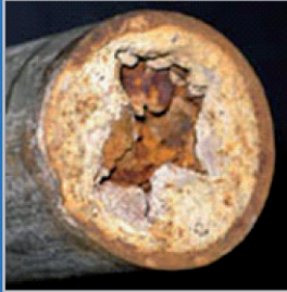
blocked pipe caused by biofilm
